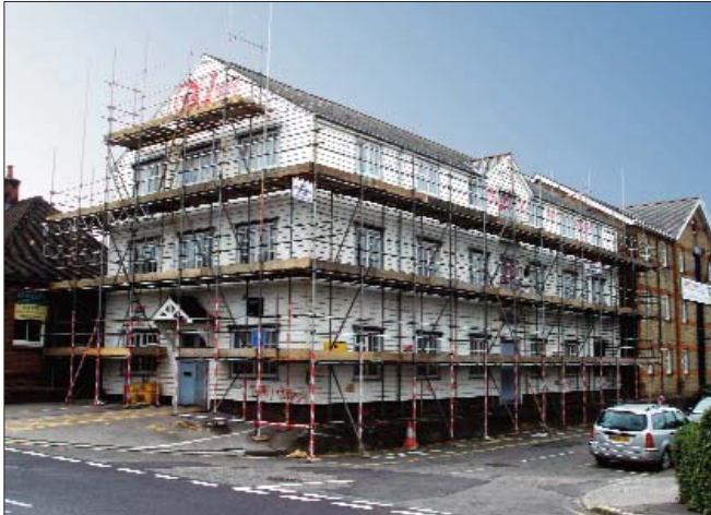
Mill House: police had to be called about the additional graffiti provided over the last week: the scaffolding evidently proved too tempting for some of the locals.
